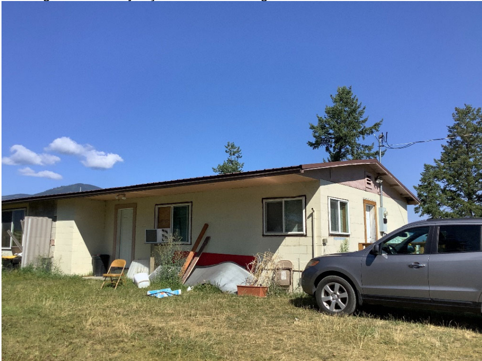
Figure 8. Detail of eaves, 147 Trading Post Road. Oblique view of south and east facing façades.
