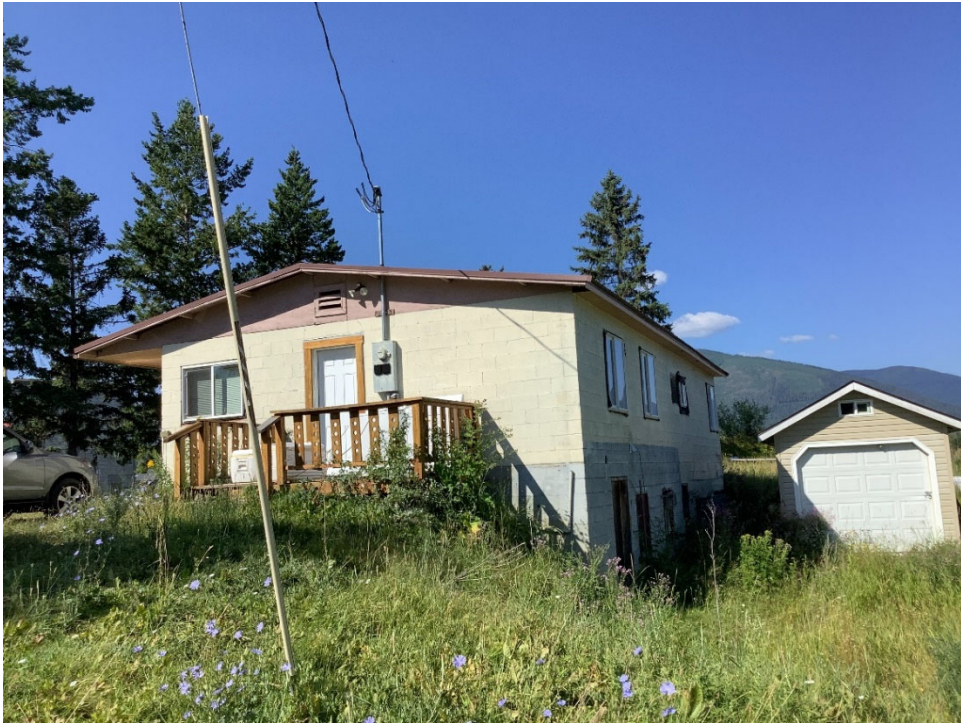
Figure 10. Detail of basement concrete block area of 147 Trading Post Road. Oblique view of east and north facing façades. View toward southwest.
