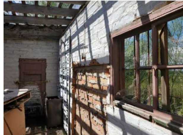
Interior of Cattle Operation Building
