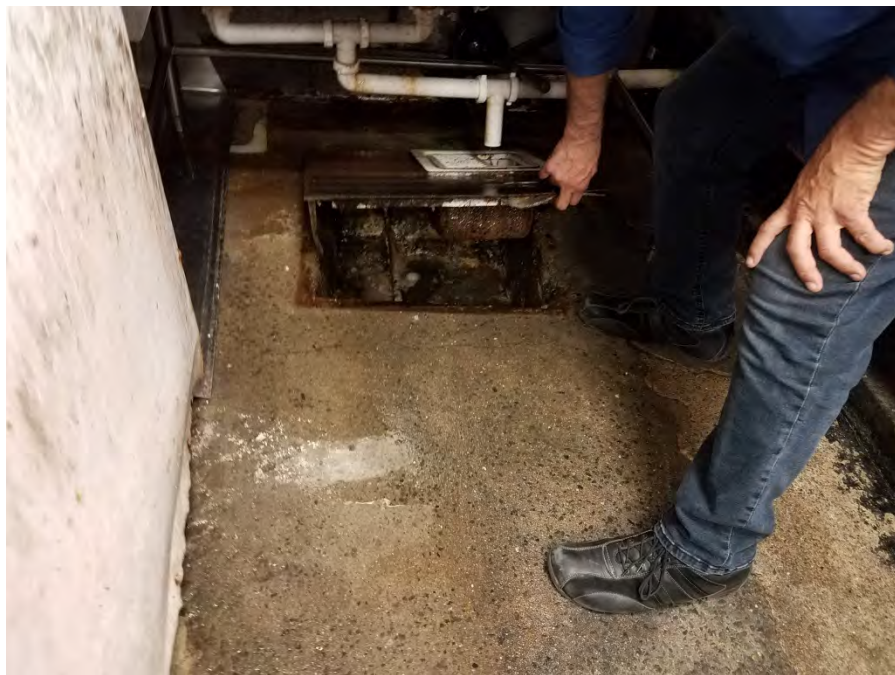
Photograph 14: View of sink drain at the meat department of the Mercado International 88 suite (747 E. San Ysidro Boulevard).
