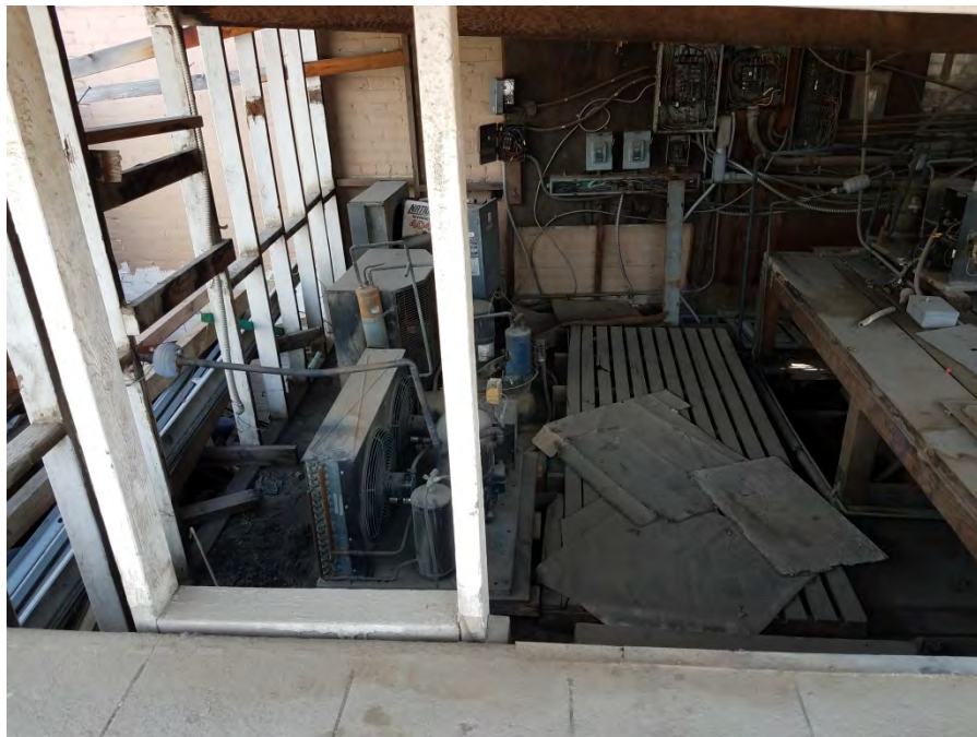
Photograph 18: Chiller enclosure on the roof of the 747 E. San Ysidro Boulevard building.
