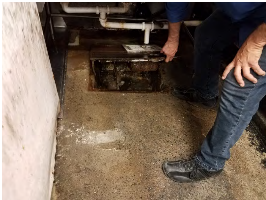
Photograph 14: View of sink drain at the meat department of the Mercado International 88 suite (747 E. San Ysidro Boulevard).
