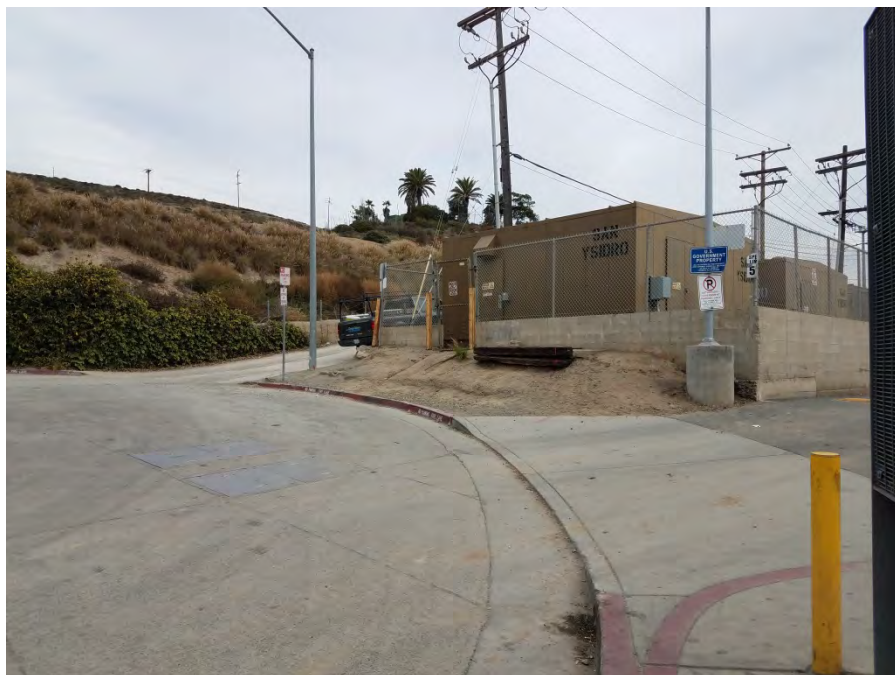
Photograph 20: View to the northeast of the site of electrical transformers.
