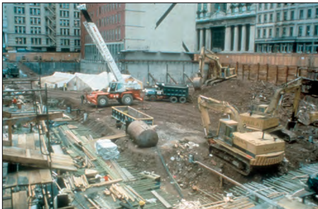
Figure 6. Construction of the 290 Broadway Federal building during archaeological fieldwork; the archaeological excavation shelter is visible at the rear. The view is toward the southeast (photograph by Dennis Seckler).
