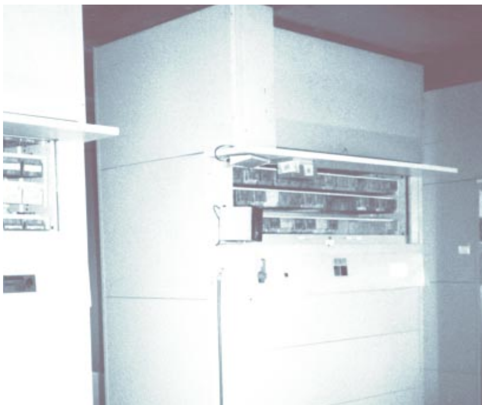
High Density Storage Unit NAS Atlanta, Marietta, GA
